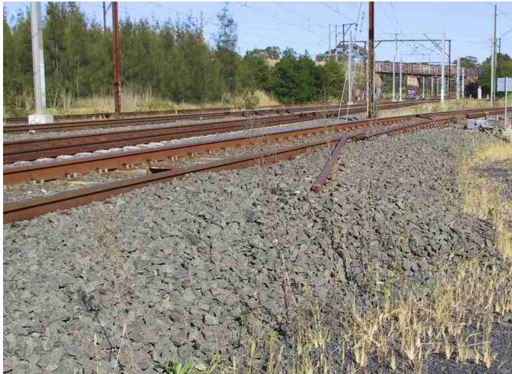
Figure 3 – Example of catchpoint with poor landing zone
