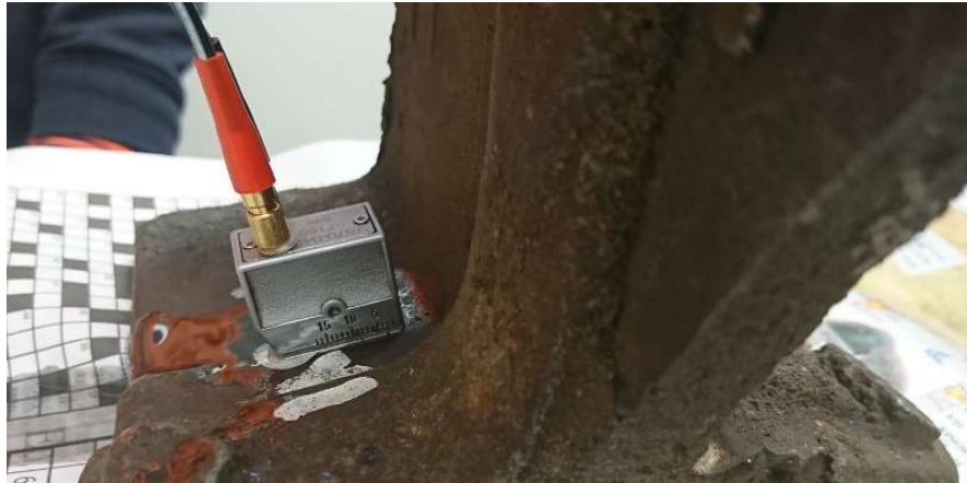
Figure 7 – Miniature 70 prob aimed across the rail foot as function check (note this is not the orientation of probe for weld foot check)
